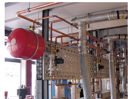
OSZ VT heating engineering laboratory and practice wall installation
